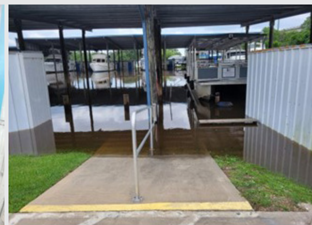
As the floor water level rises, the boat floats high in the stall and the storage units are taking on water. All school supplies, boat equipment, and PFD's have been moved to safety.
